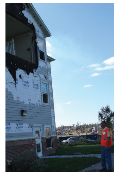
MSPE President Kurt Higgins observes damage to a structure in Joplin.
